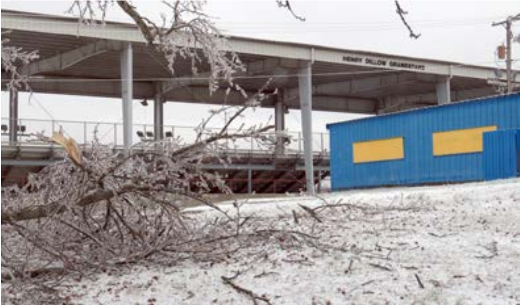
Fallen tree limbs coated in ice were on the ground Tuesday, Jan. 7, near the Henry Dillow Grandstand and the Anna Kiwanis Club building at the Anna City Park.
